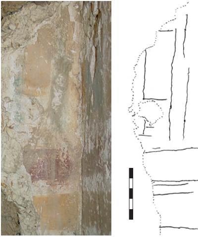
Fig. 34a-b The only remains of the decoration of the rear wall: dado and vertical block border in the north-east corner.
